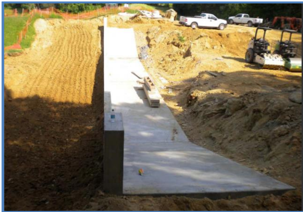
Photo shows construction of one of two concrete cutoff walls in the auxiliary spillway.
