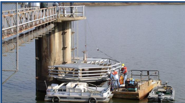
Rehabilitation included raising the height of the dam and the elevation of the principal spillway inlet.
