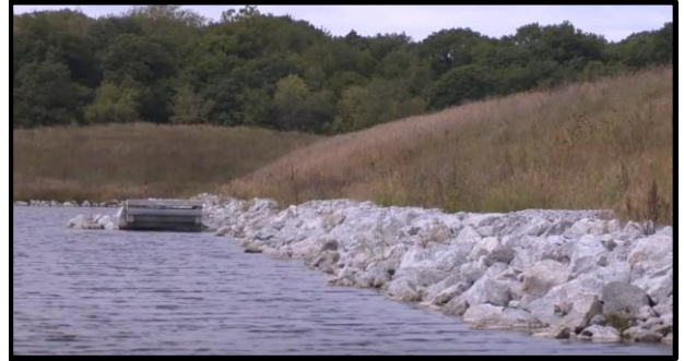
The Duck Creek dam was constructed in 2016 for flood protection and recreation.
