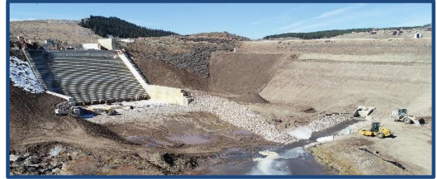
A new concrete labyrinth spillway was installed as part of the rehabilitation project.
