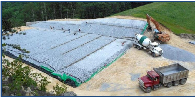
The rehabilitation of the dam included armoring the auxiliary spillway with concrete blocks that are cabled together.
