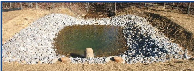
A riprap stilling basin replaced a concrete box at the outlet of the principal spillway pipe.
