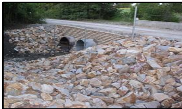
A completed sand cement bag riprap wall with rock riprap chutes in Texas protects bridge and road.
